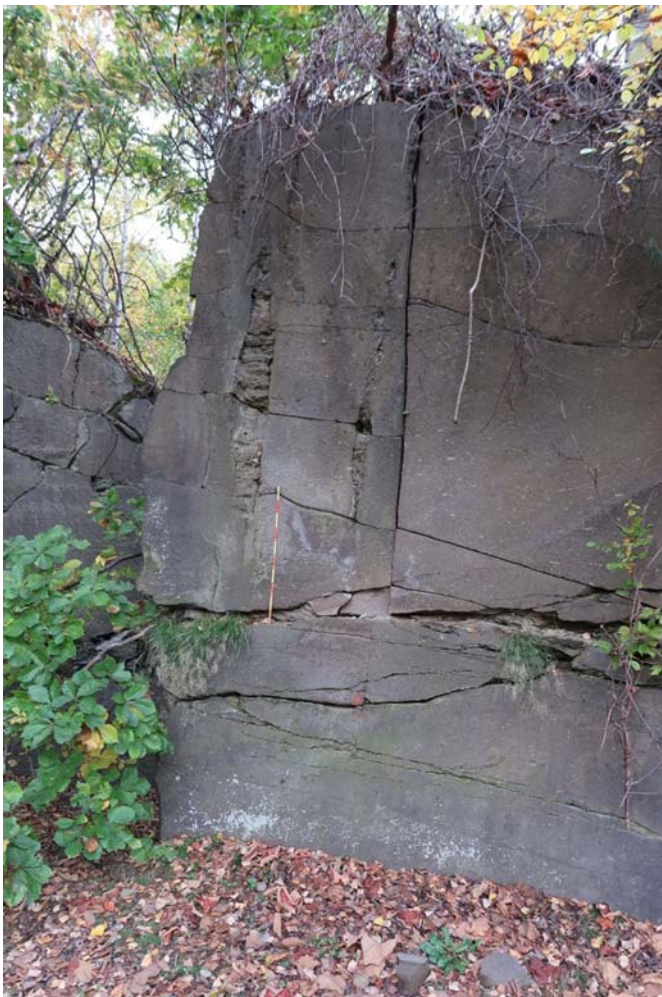
写真-9 溶結凝灰岩に鉛直に
